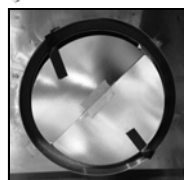
Black Tape on Damper
